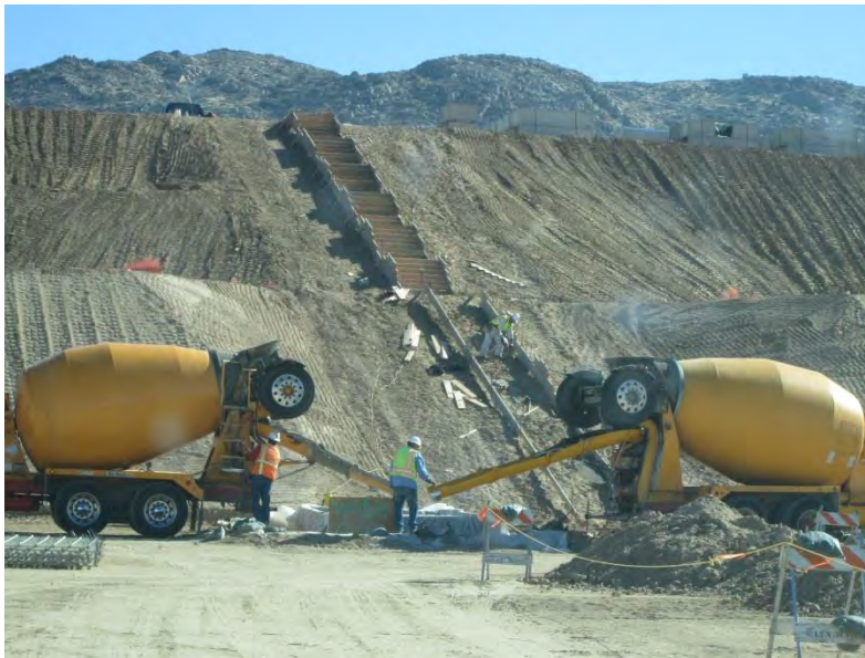
Photo 8: A concrete washout is utilized by cement truck operators to wash equipment prior to leaving the right-of-way in accordance with the SWPPP and MM-HYD-1.
