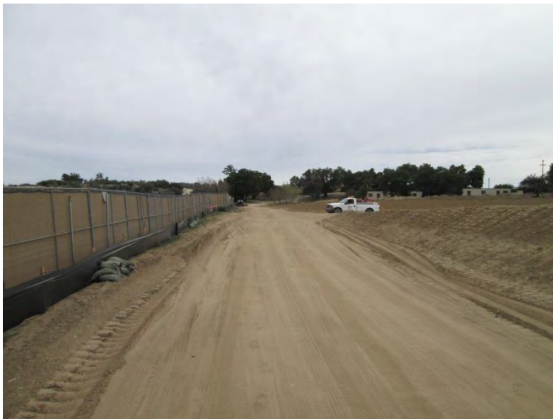
Photo 2: In accordance with the Construction Fire Prevention Plan (Mitigation Measure FF-1), a fire watch is present at the Boulevard Substation during construction.
