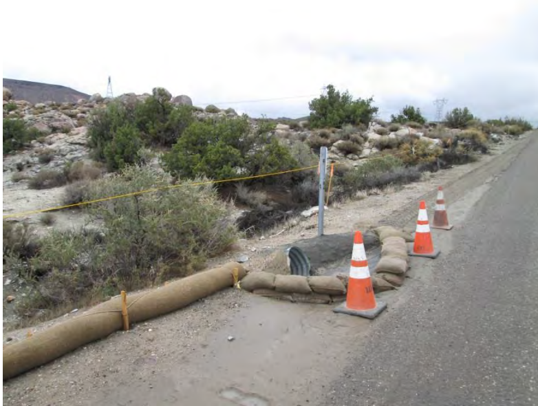
Photo 3: BMP's were observed in place prior to construction activities associated with the 138 kV underground being initiated along Old Highway 80. Gravel bags and straw wattles can be seen in this photo to minimize the potential for pollutants and sediment to enter into a storm drain located along Old Highway 80.
