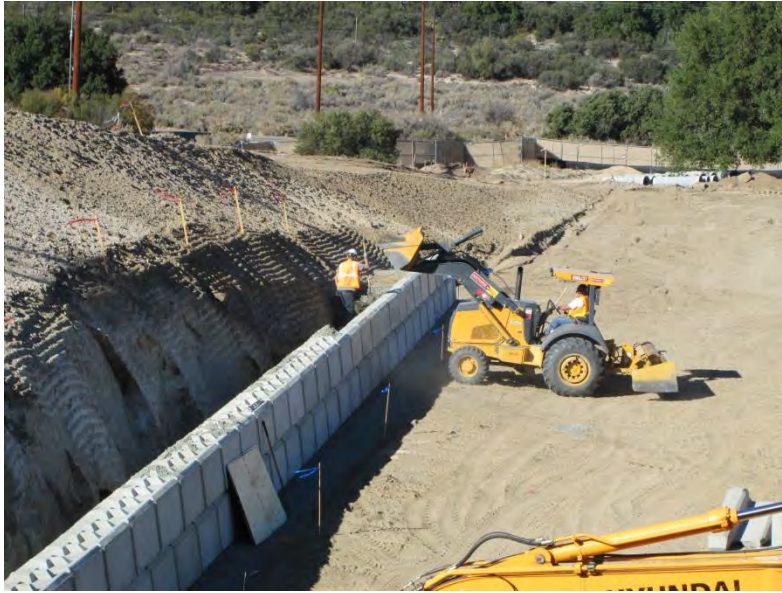
Photo 1: Construction activities associated with building a retaining wall along the western limits of the Boulevard Substation were initiated during this reporting period.
