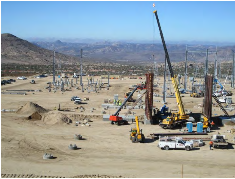
Photo 7: An overview of the ECO substation construction looking west towards the 138/230 kV pad. A crew can be seen in the forefront of the photo utilizing a crane to construct fire walls that will be located on either side of a transformer.
