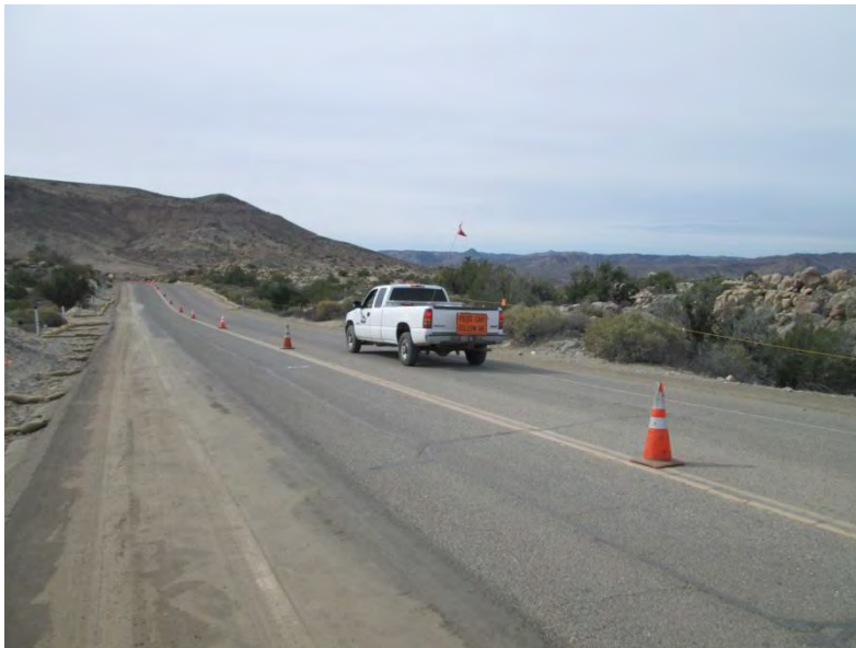
Photo 4: Construction activities required traffic to be reduced to one lane resulting in the need for an escort car to be utilized for both eastbound and westbound traffic along Old Highway 80. Traffic control measures were observed being implemented as required in the Traffic Control Plan and MM-TRA-1.
