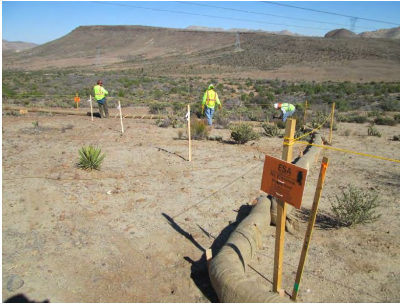
Photo 5: Construction crews were observed placing BMP's at overhead transmission line pad sites in accordance with MM-HYD-1 and the SWPPP. Signage was also observed being placed adjacent to Environmentally Sensitive Areas along the right-of-way as required in MM-CUL-1a.
